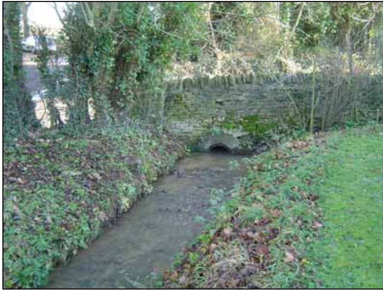
Downstream face of Shipton Road culvert carrying Coldwell Brook in the grounds of Coldwell House
