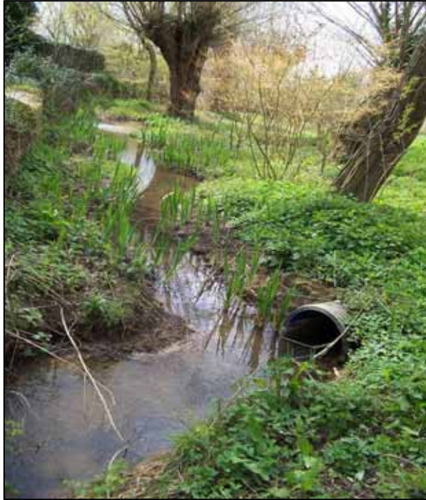
Coldwell Brook downstream of Coldwell House looking downstream towards R.Eventlode showing location of drainage outfalls and condition of channel
