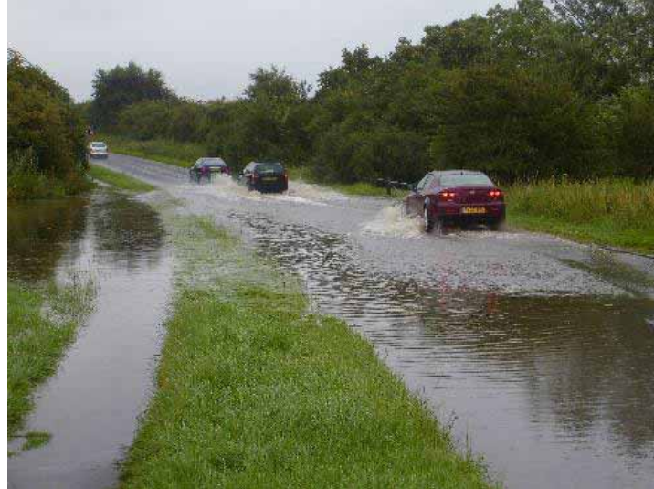
Flooding July 2007 - Flooding on Bampton Road (A4095), Curbridge where Elm Bank Ditch flows beneath Bampton Road.
