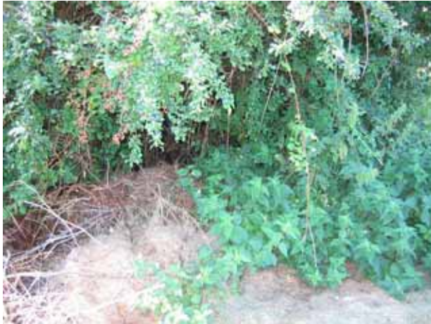
Area 1 – Blocked drain at Witney Road west
