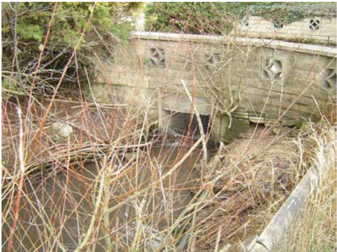
Area 2 – Northmoor Village Choked village brookcourse culvert to be cleared out and culvert upsized
