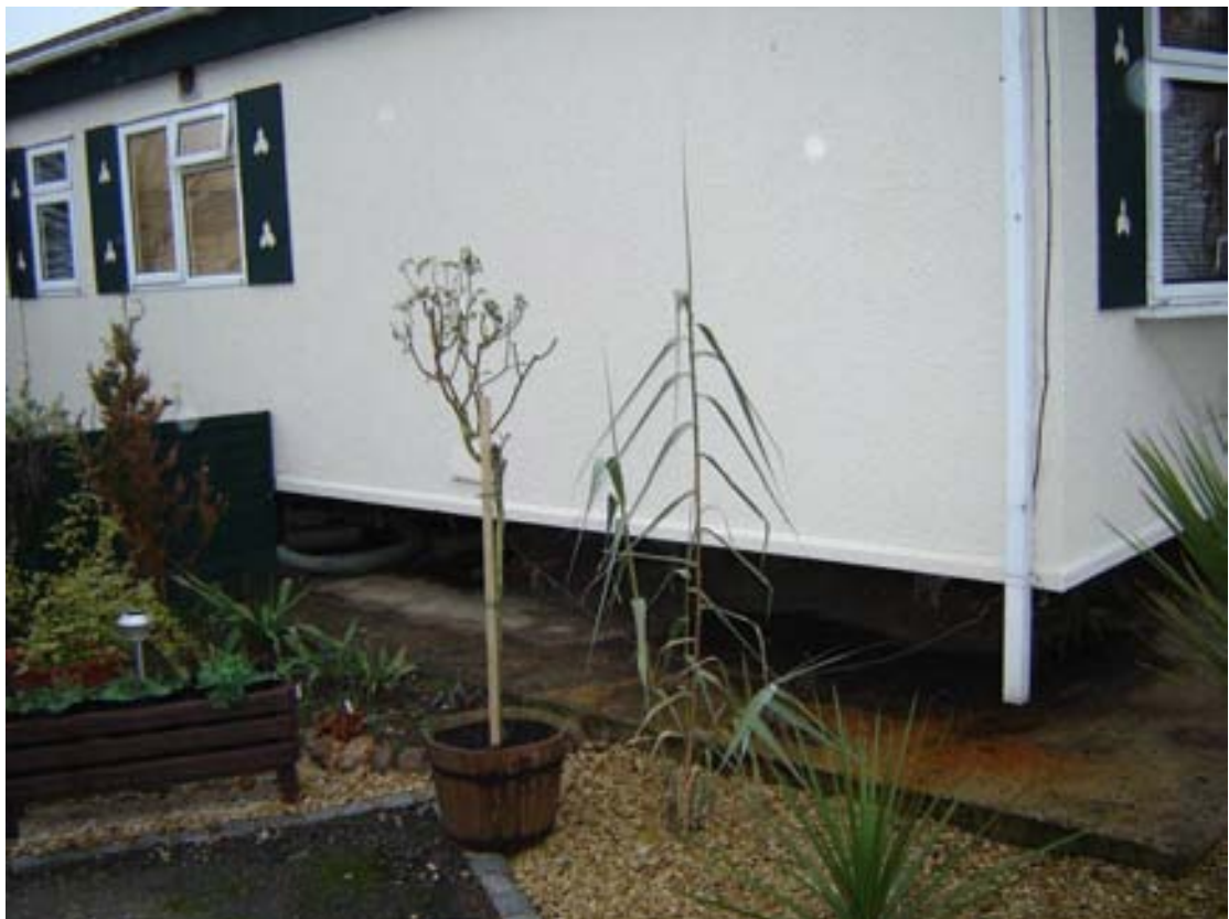
Area 1 – Bablock Hythe Caravan at Thameside Caravan Park jacked up by 300mm
