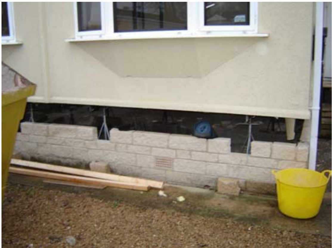
Area I – Bablock Hythe Caravan at Thameside Caravan Park jacked up by 300mm
