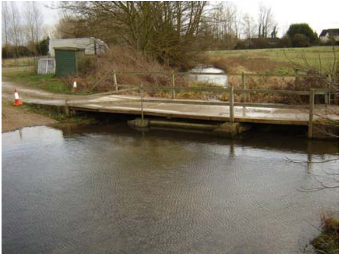
Area 2 – Northmoor Village Overgrown village brookcourse at Pinnocks Farm requiring cleaning out
