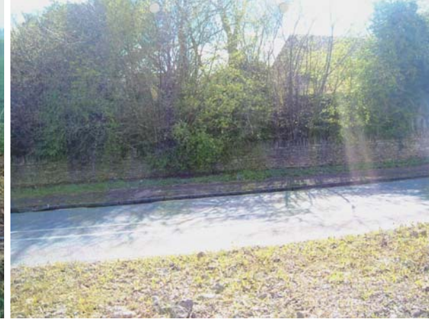
Area 4 - Kerb damage, due to ponding water on highway
