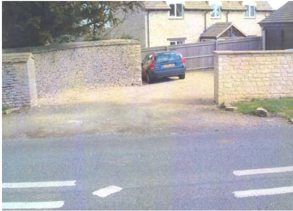
Area 1- No kerb face on driveway
