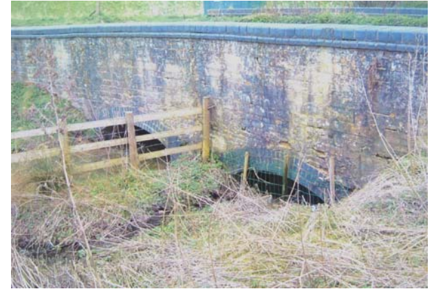
Area 2- Partially blocked arches at bridge on B4030
