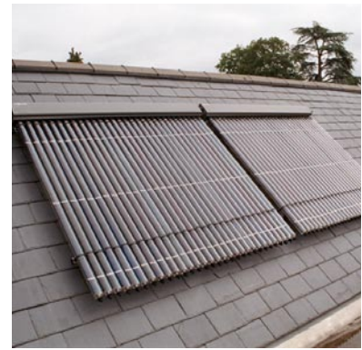
Fig. 28 Solar thermal panels - evacuated tube type
