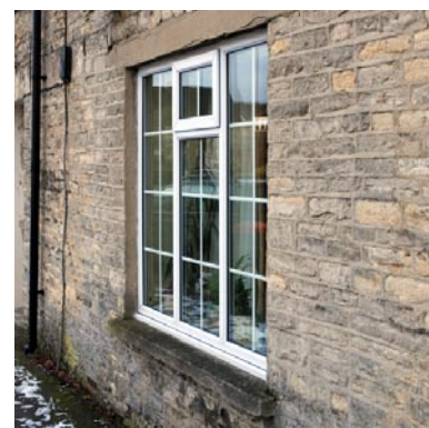
Fig. 17 Visually harmful double-glazing with sandwiched glazing bars
