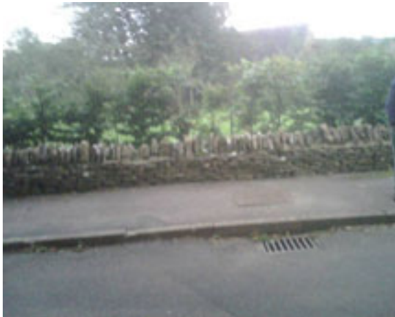
Point looking downstream, at direction of culverted watercourse, towards property in Chapel Close
