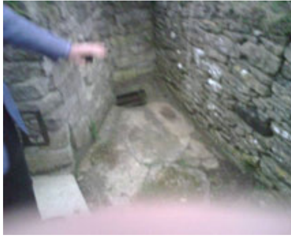
Open grille on culverted watercourse, which passes through private property in Chapel Lane
