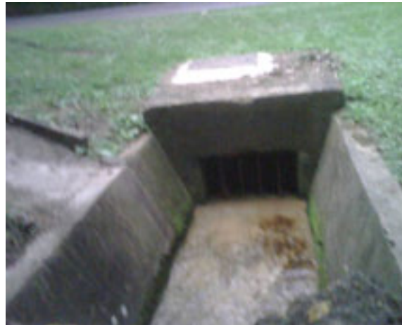
Vertical grating, which receives highway drainage and land drainage run-off
