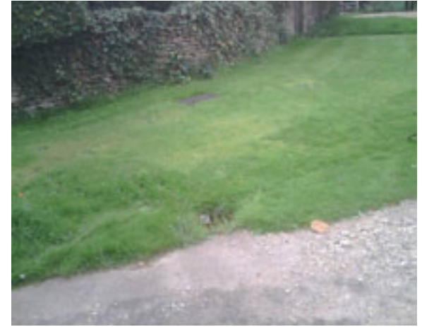
Manhole on culverted watercourse and position of highway gully connected to it
