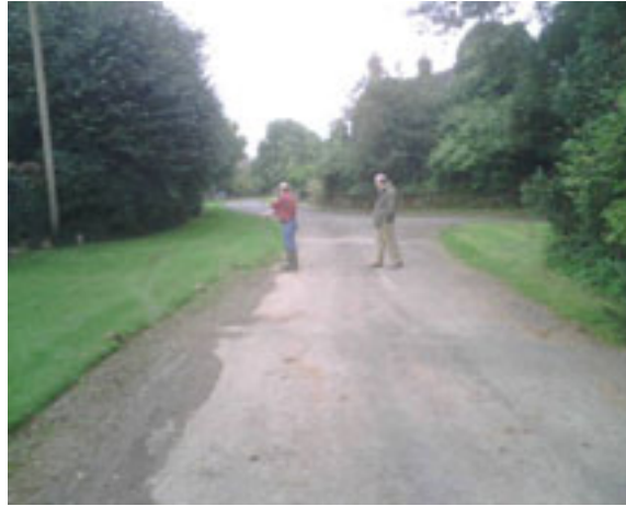
Position of blocked / broken highway gully and soakaway at The Green
