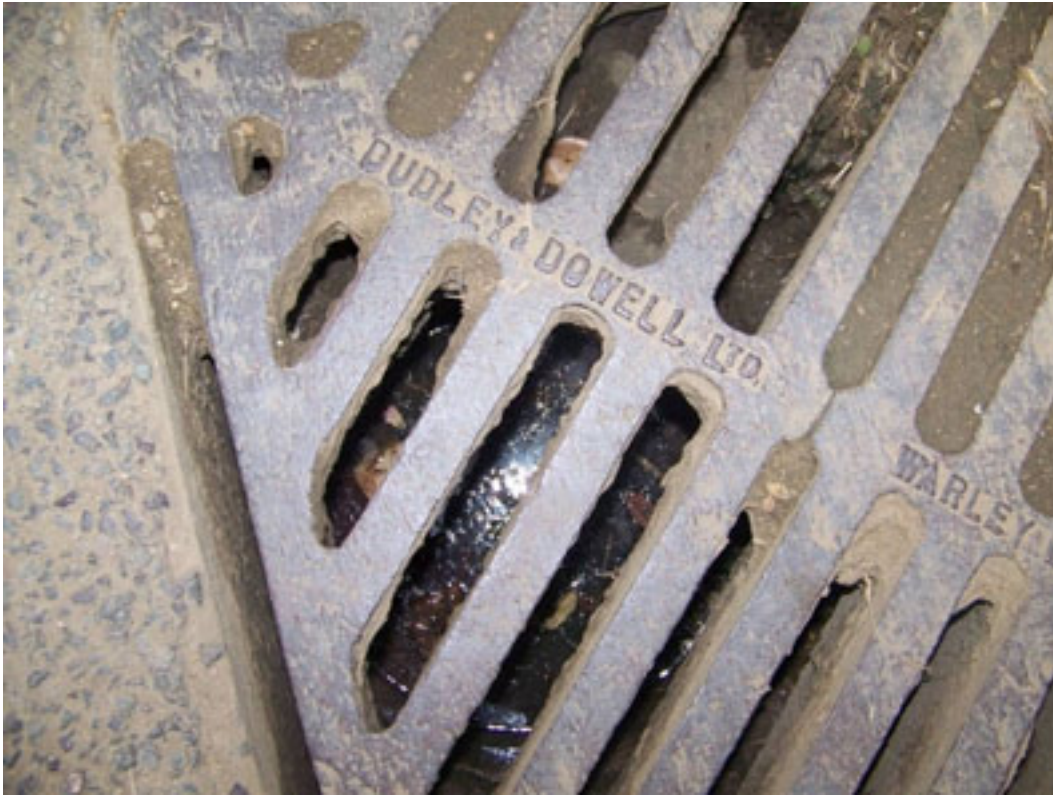
Blocked gully pot – Lechlade Road
